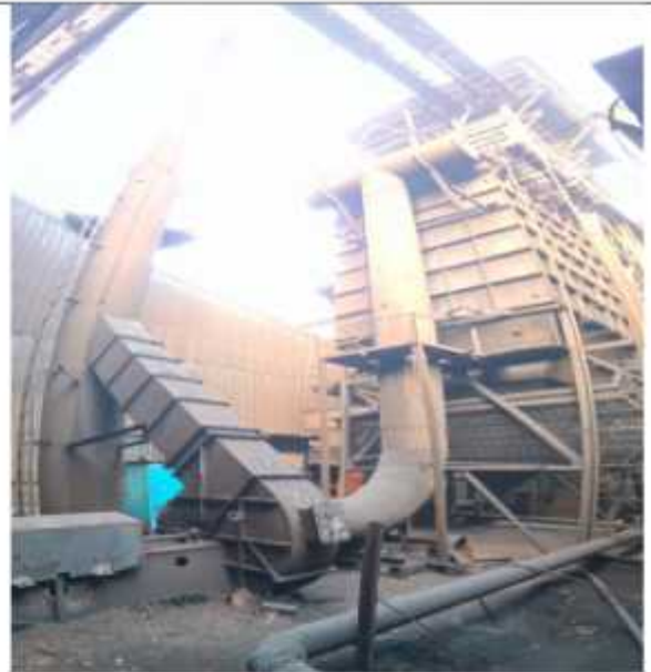
Bag Filter Connected with 5 × 20 T Induction Furnace
